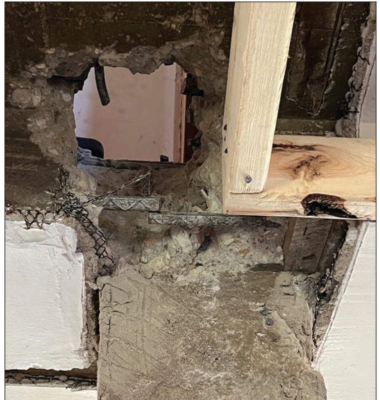
The hole in the floor, beam, and column damage that were discovered during renovations.
