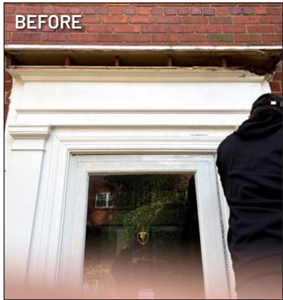
938/3522 Valley Drive, Damaged Trim Replacement
