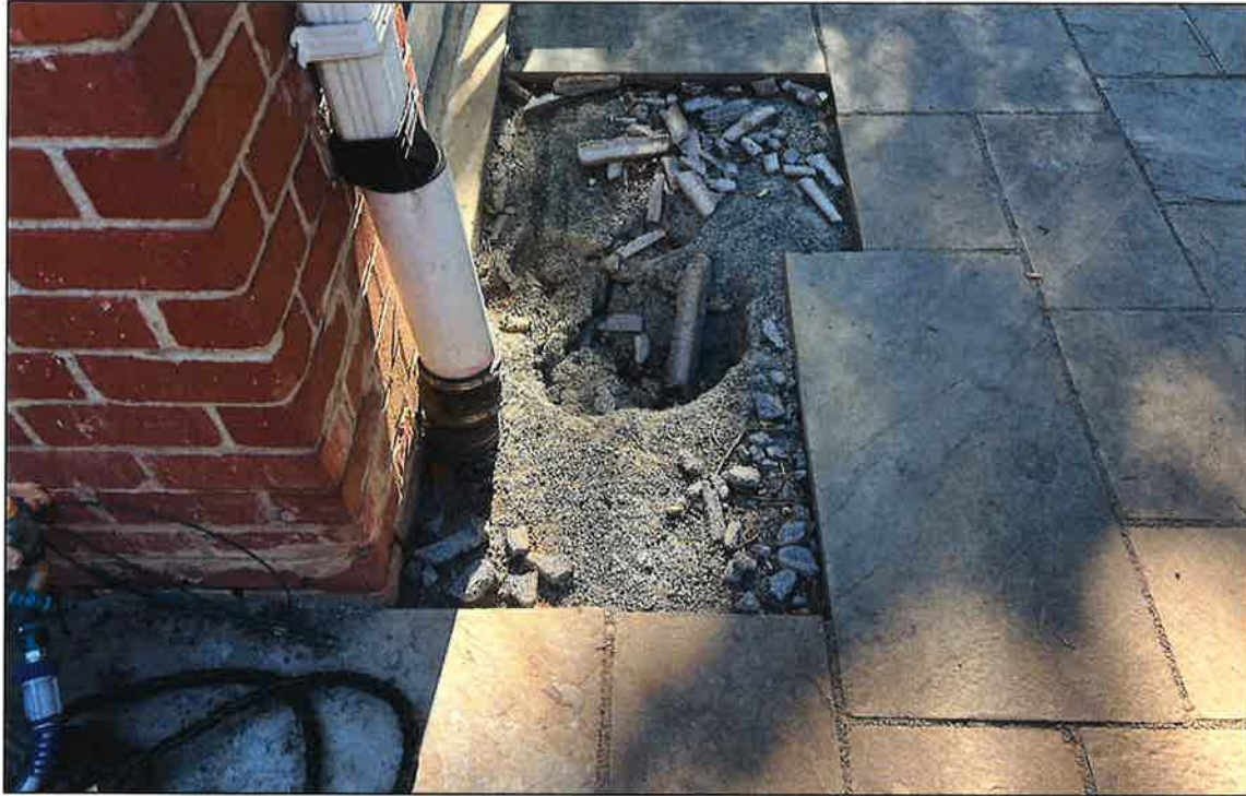
Photo 4. Rear porch of Unit 1670 sinking towards the building.
