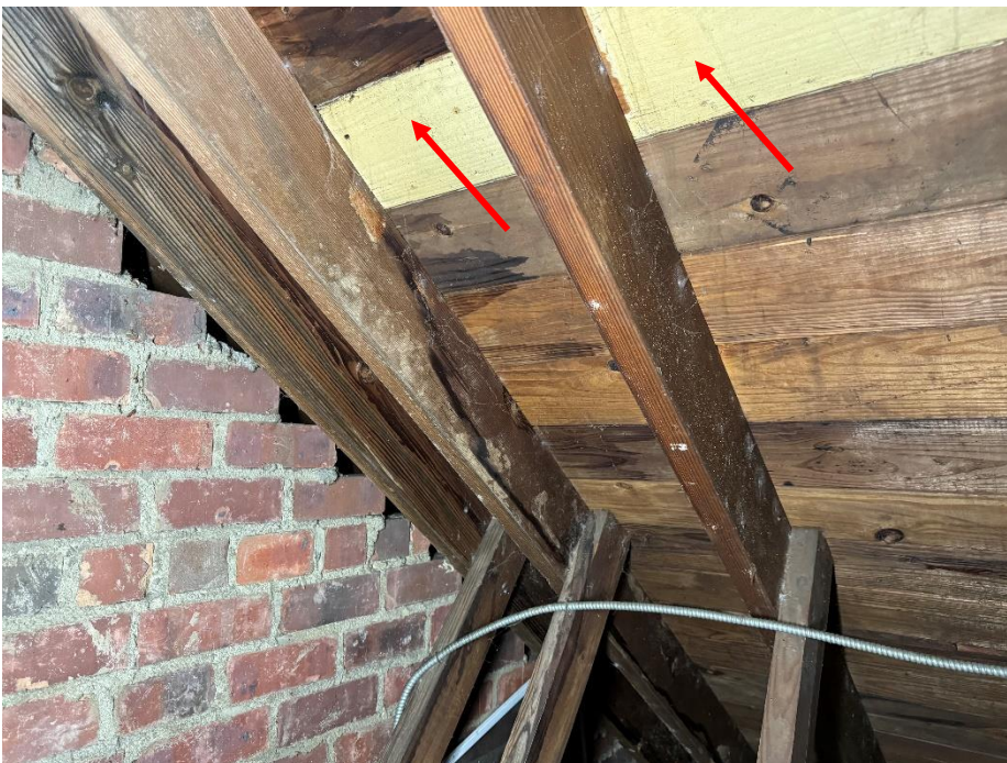
Photo 20. Bldg. 403 – Unit 1427: Red arrows pointing to coating applied on roof sheathing. Evidence of moisture intrusion on roof truss adjacent to applied coating.
