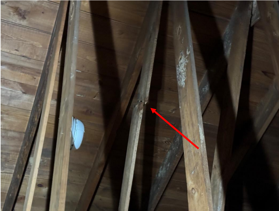
Photo 7. Bldg. 827 – Unit 3331: Red arrow pointing to broken web chord of roof truss.
