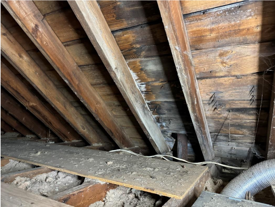
Photo 13. Bldg. 849 – Unit 3229: Step away of region where white staining was observed.
