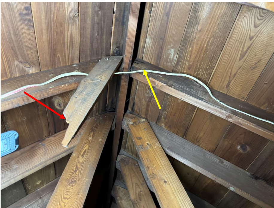
Photo 8. Bldg. 953 – Unit 1500: Red arrow pointing to damaged web chord of roof truss. Yellow arrow pointing to missing web chord of roof truss.
