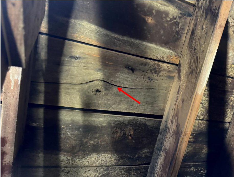
Photo 5. Bldg. 510 – Unit 3714: Red arrow pointing to crack in roof sheathing.
