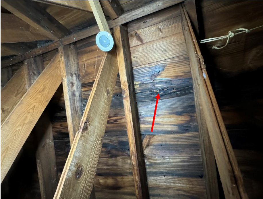
Photo 15. Bldg. 849 – Unit 3229: Red arrow pointing to deteriorated roof sheathing.
