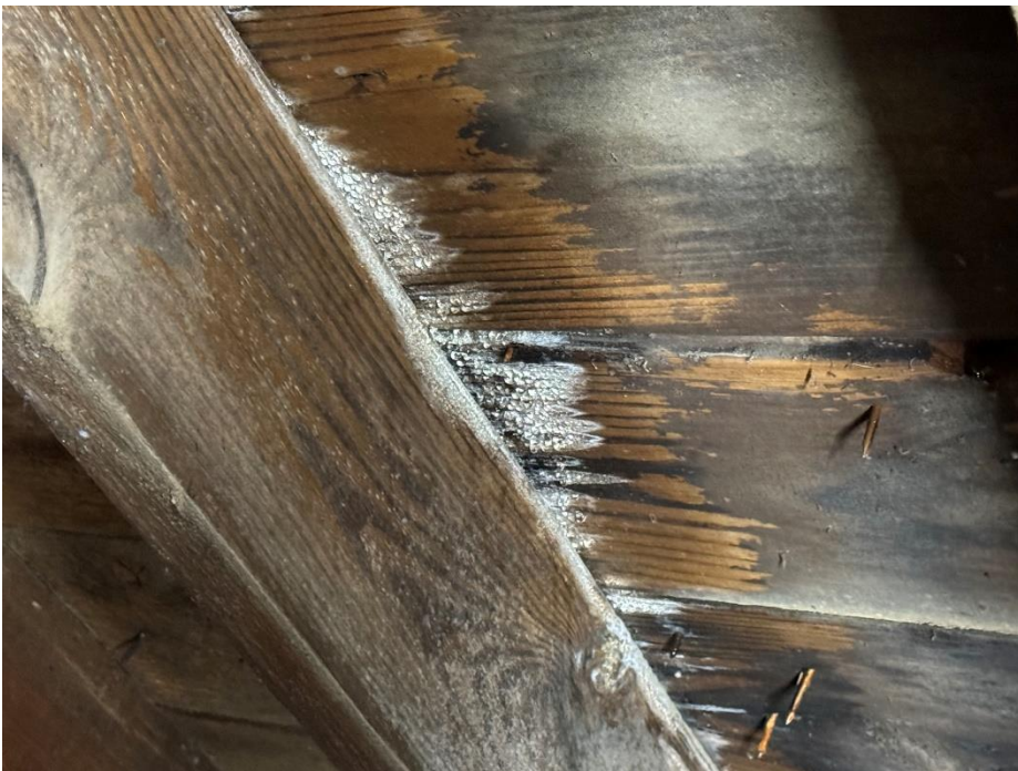
Photo 14. Bldg. 849 – Unit 3229: Moisture observed where white staining was encountered.
