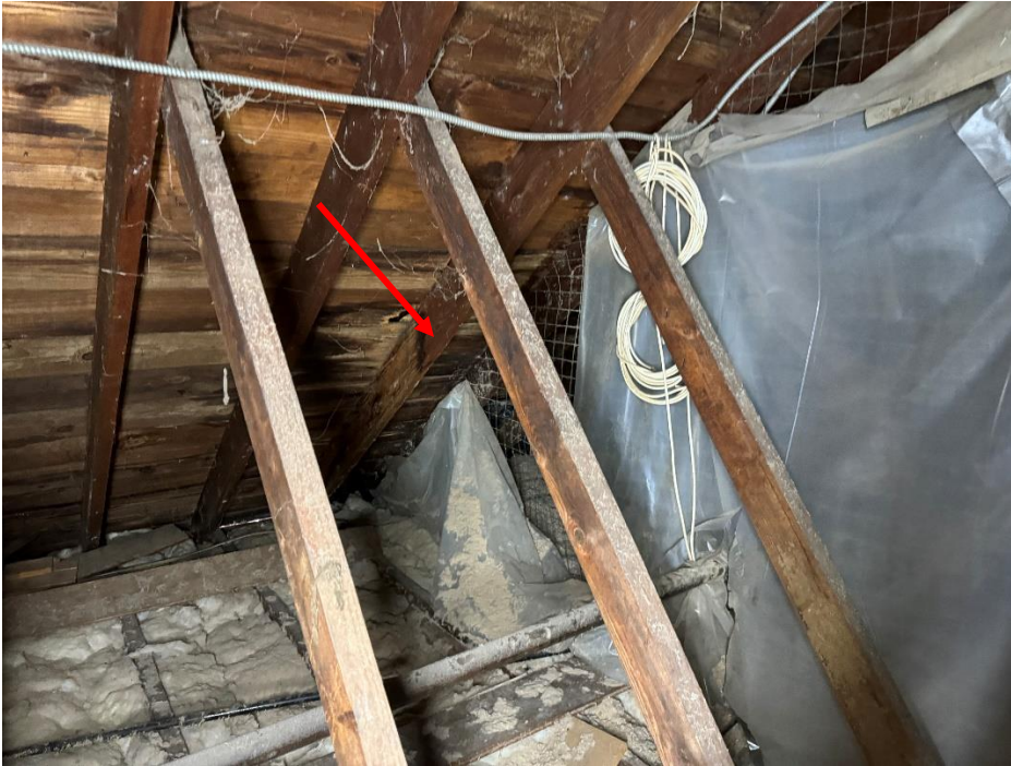
Photo 11. Bldg. 403 – Unit 1429: Red arrow pointing to section loss in roof sheathing.
