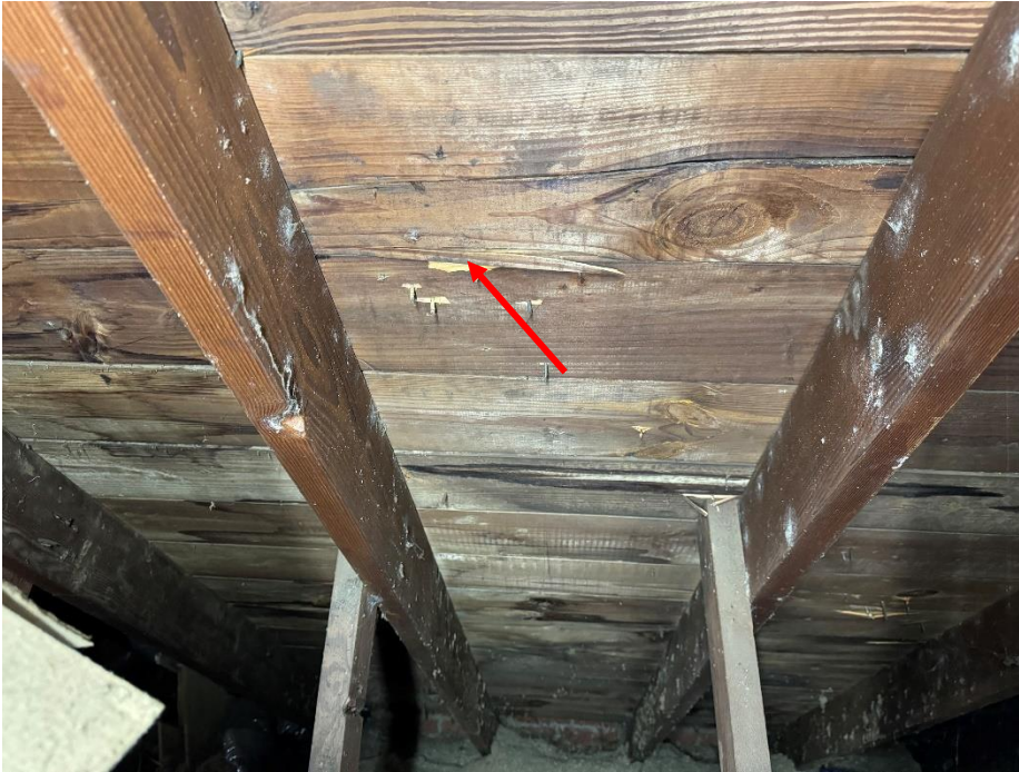
Photo 19. Bldg. 403 – Unit 1427: Red arrow pointing to crack in roof sheathing.
