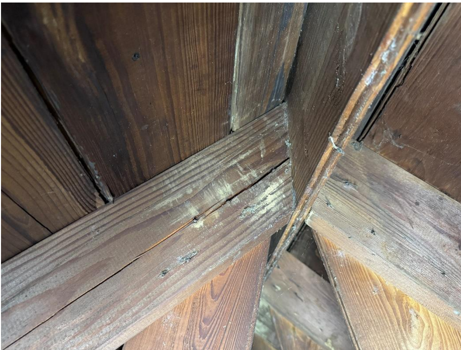
Photo 6. Bldg. 403 – Unit 1427: Top chord of roof truss with split.
