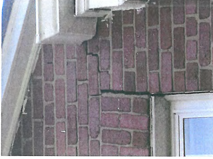
32. Bldg 723: Step crack at rear façade (potentially exacerbated by August 5, 2010 storm/tree fall damage).
