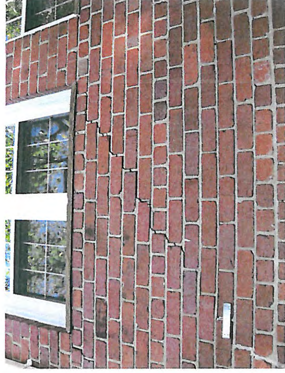
8. Bldg 838: Step crack and masonry separation at rear elevation of Unit 3227.
