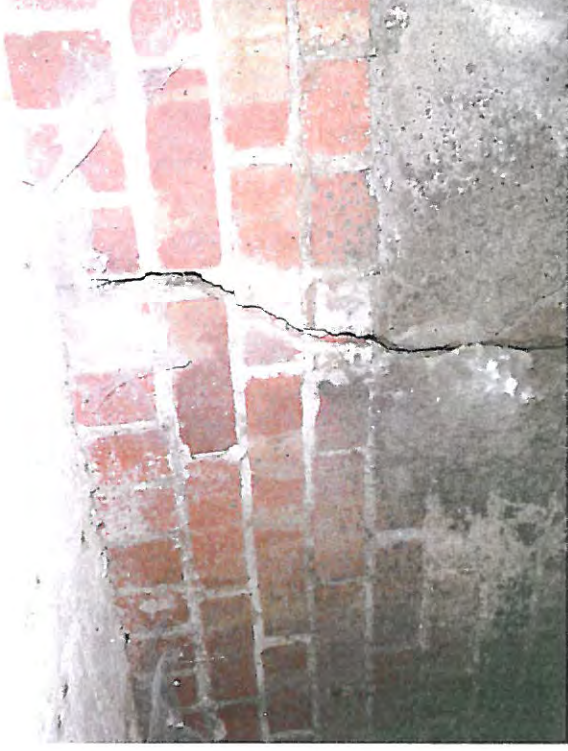
23. Bldg 718: Step crack and horizontal separation at foundation wall (as viewed from crawl space).
