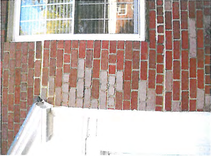
12. Bldg 111: Rotation at masonry pier at front elevation.
