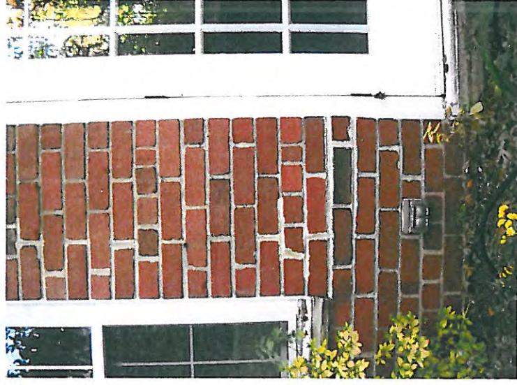
29. Bldg 112: Rotation at masonry pier at rear elevation.
