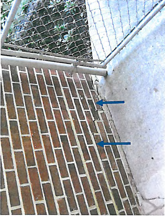
25. Pool Bldg A: Step crack with substantial separation at breezeway front corner.
