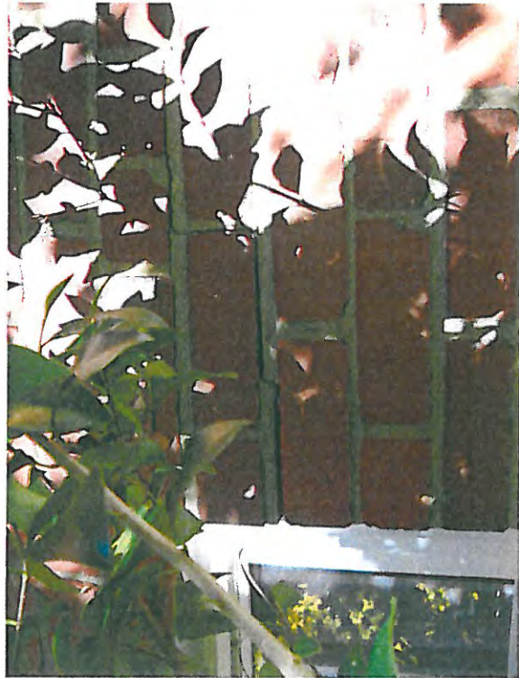
19. Bldg 537: Separation and rotation at masonry pier at Unit 3718 (Rear elevation).
