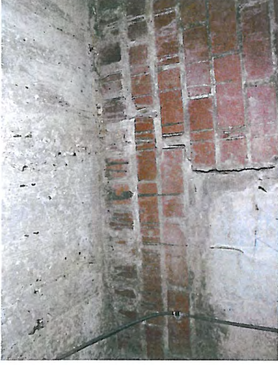
22. Bldg 718: Step crack/separation at foundation wall (as viewed from crawl space).
