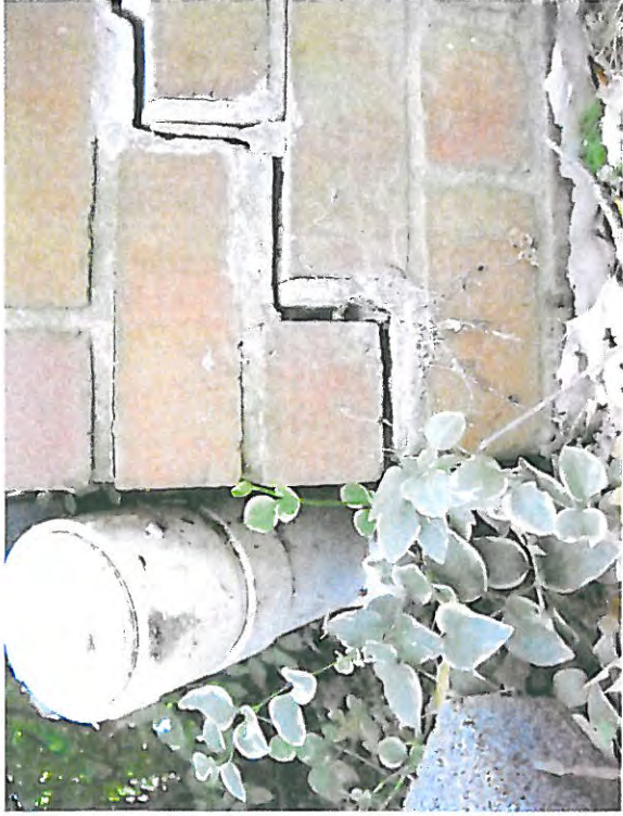
5. Bldg 830: Horizontal displacement at front corner of Unit 3133 (Side elevation).
