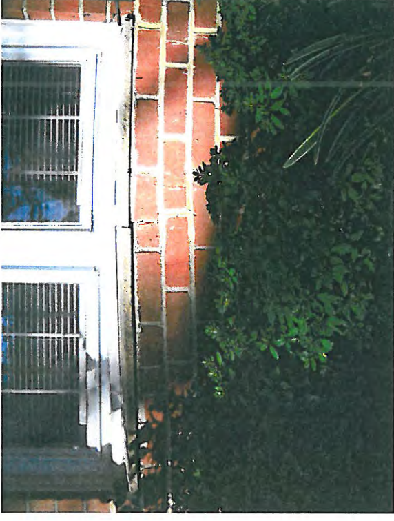
10. Bldg 111: Window sill rotation at front elevation.
