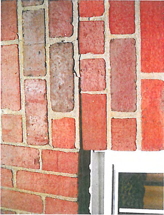
18. Bldg 537: Separation and rotation at masonry pier at Unit 3718 (Rear elevation).
