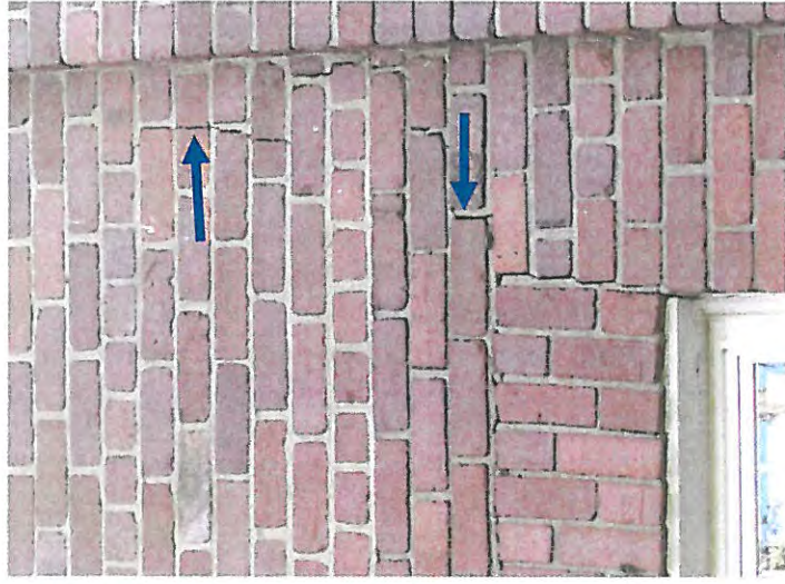
33. Bldg 723: Step crack at rear façade (potentially exacerbated by August 5, 2010 storm/tree fall damage).
