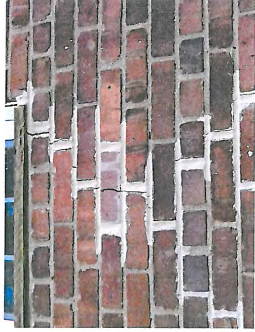
17. Bldg 716: Step crack at previously repaired masonry at rear elevation.
