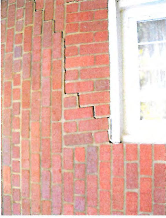
6. Bldg 830: Step crack at masonry lintel of Unit 3133 (Side elevation).
