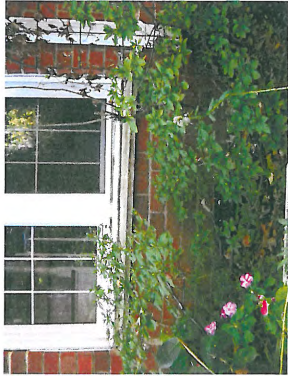
28. Bldg 112: Window sill rotation at rear elevation.
