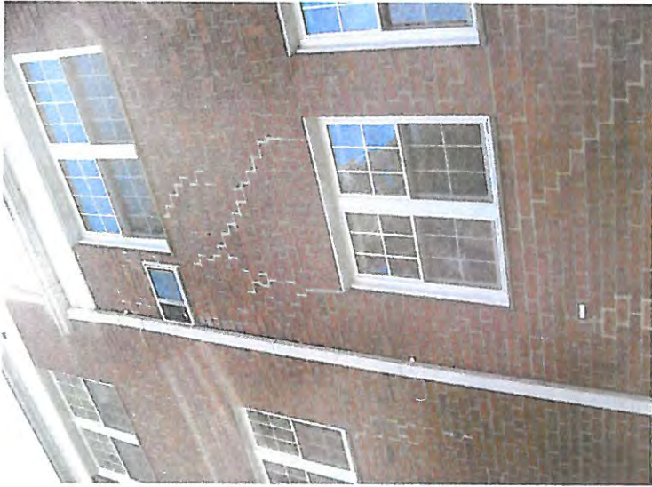
24. Bldg 718: Evidence of several masonry repairs throughout rear elevation.
