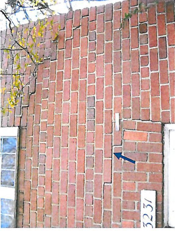
2. Bldg 849: Step crack at rear corner of Unit 3231 (Rear elevation).
