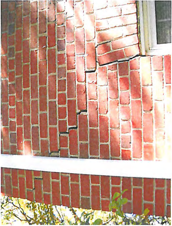
1. Bldg 849: Step crack at rear corner of Unit 3231 (Side elevation).
