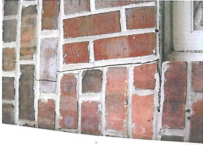
15. Bldg 716: Crack at previously repaired masonry at rear corner of Unit 3210 (Rear elevation).
