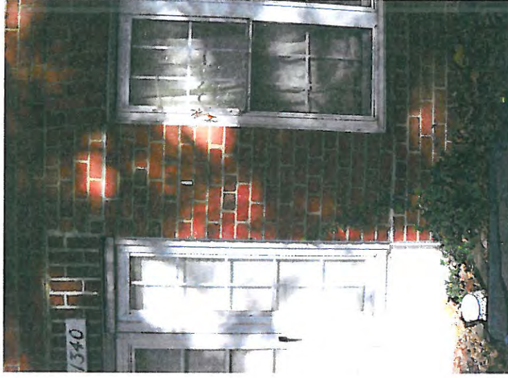
20. Bldg 527: Rotation at masonry pier at Unit 1340 (Rear elevation).
