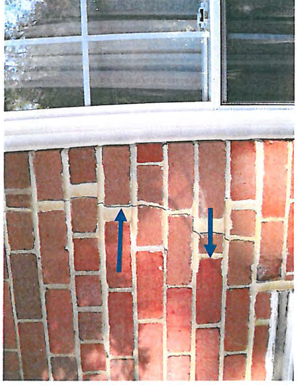
11. Bldg 111: Crack at previously repaired masonry at rear elevation.
