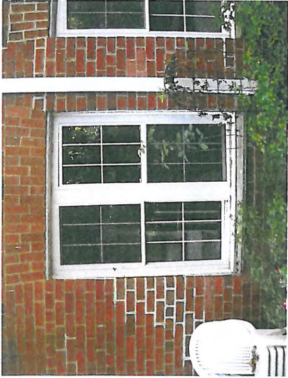
30. Bldg 112: Displacement (racking) of window assembly at rear elevation.
