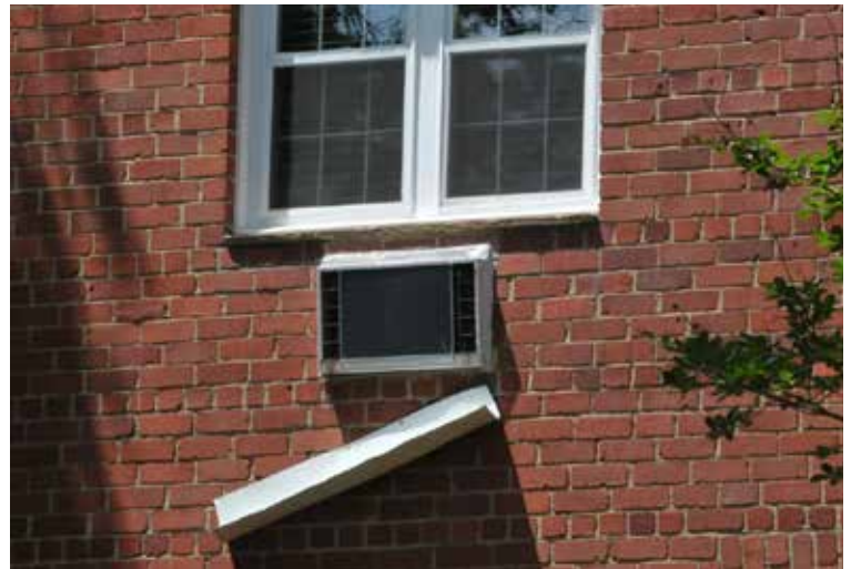
A metal diverter shown under an air conditioning unit.
