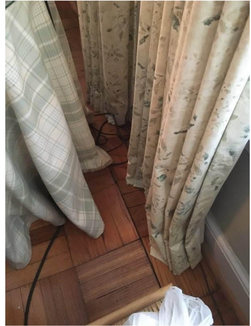
Tiles buckled Feb 2020
